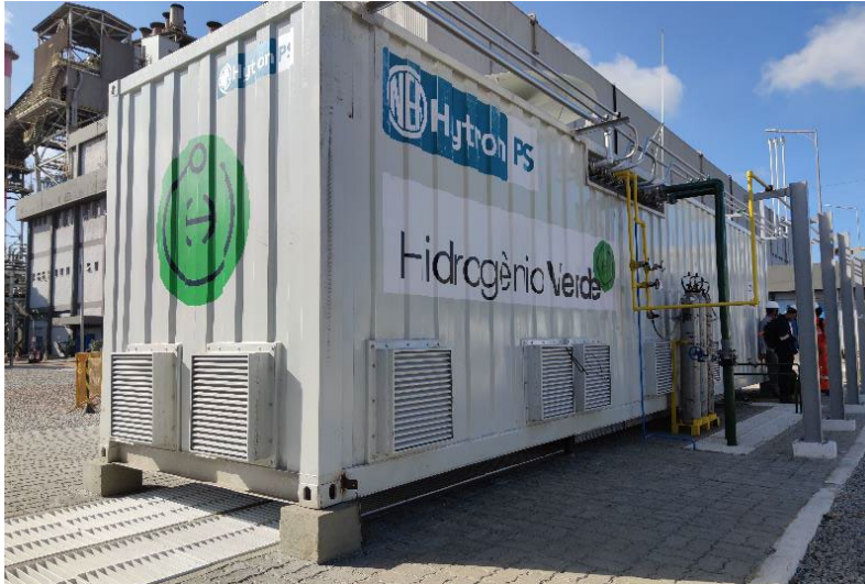
1.3 MW Electrolyzer System Fortaleza, Brazil
