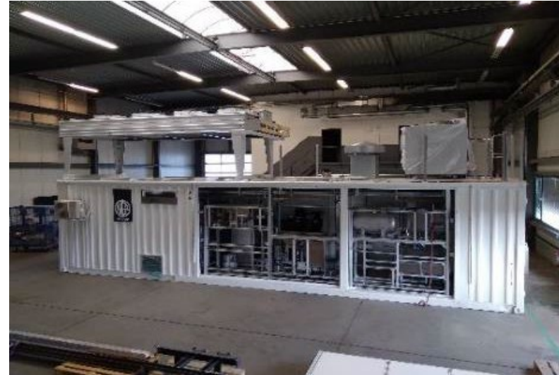
1.0 MW Electrolyzer System Bavaria, Germany
